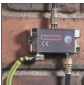
ESP CATV/F installed in a basement or garage near where the coaxial cable enters the building
