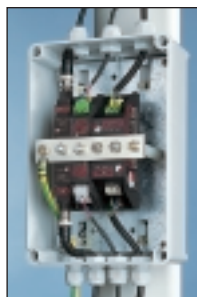
Protectors for the video (ESP CCTV/B, left), camera telemetry (ESP 15E, centre) and the low current mains power (ESP 240-5A, right) inputs to a camera, installed together on a CME 4 mounting and earthing kit. Note that the protectors have been cross bonded to the metal work of the pole (out of shot).
