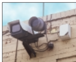
CCTV camera protected from a direct lightning strike, by one of the building's 'lightning conductors', and from transient overvoltages by protectors in a WBX 4/GS secure enclosure.
