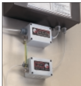
Security alarm panel with ESP TN/BX (bottom) providing protection from transient overvoltages on the dial-up telephone line. Note how the ESP TN/BX is earthed via a bond to the ESP 240-16A/BX (top) installed on the mains power supply to the panel.
