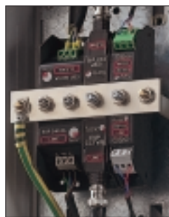
To protect an outside CCTV camera, protection on the power supply (here an ESP 240-5A) is installed alongside video and telemetry line protection, on a CME 4 (mounting and earthing kit), inside a WBX 4/GS enclosure.
