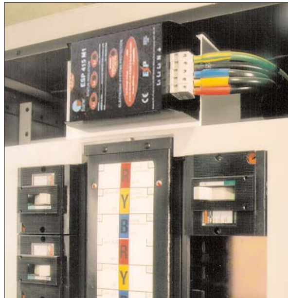
Figure 1 - ESP 415 M1 installed inside a power distribution panel.
