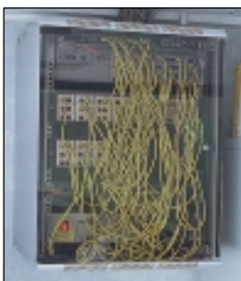
Protect hubs and other equipment from transient overvoltages on network cables from other buildings.
