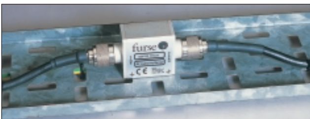
ESP RF 111A11 installed on a coaxial cable running between an antenna and an RF receiver. Note the earth lead (behind the cable tray) attached to the mounting fixture.
