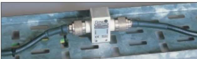
ESP RF 111121 installed on a coaxial cable running between an antenna and an RF receiver. Note the earth lead (behind the cable tray) attached to the mounting fixture.
