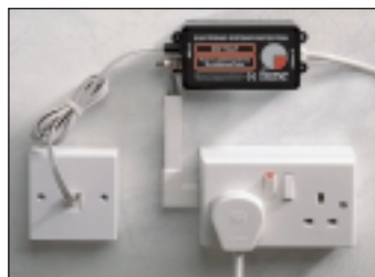
The installation above clearly shows a protector installed with a short earth connection to the same earth as the equipment it's protecting
