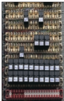
Single line protectors (here ESP KT1s) installed on LSA-PLUS disconnection modules, via ESP KE10 earth bars, to all incoming telephone lines and individual extension lines to other buildings.
