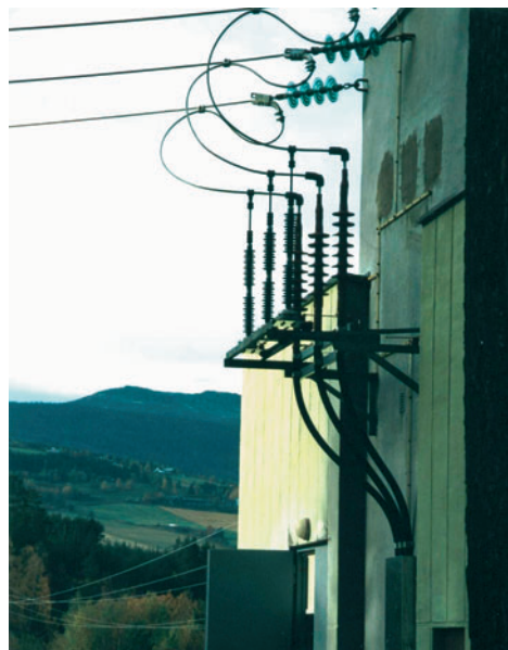
66kV Surge Arresters - Statkraft, Norway
