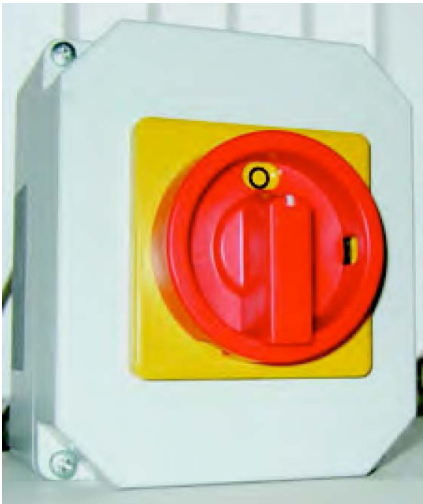
Figure 62. Main power switch
